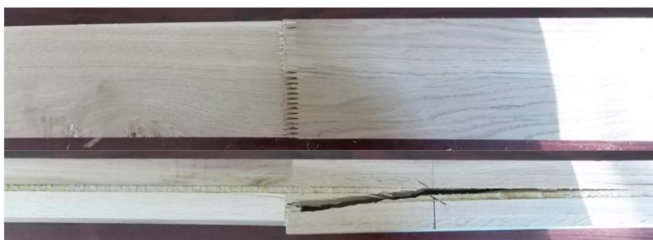
Figure 6: Pictures of a typical finger joint failure in specimen 38
